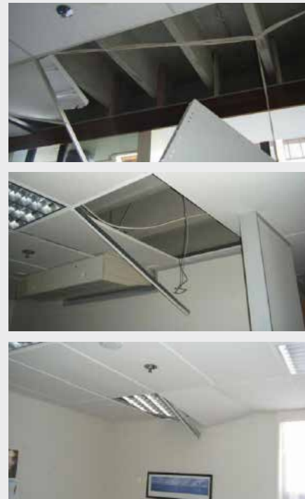
Figure 2 - Examples of damage to suspended ceilings 1
